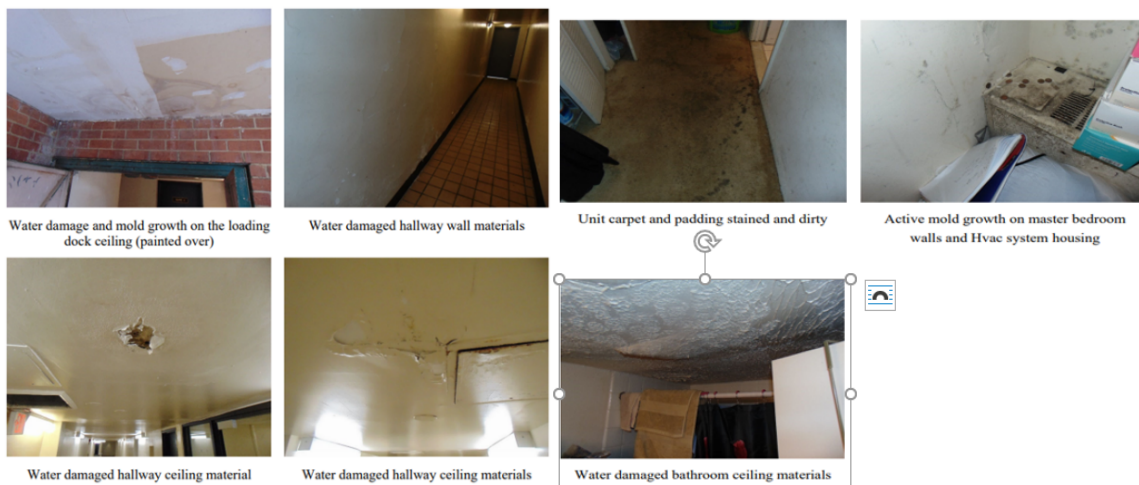
(Pictures from June 2021 Arrowhead Consulting mold inspection at Marbury Plaza)
